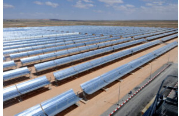
Thermo-solar power plant
