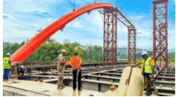
Construction of the Hawaiian Bridge on the Coastal Highway, funded by the ConnectPNG program
