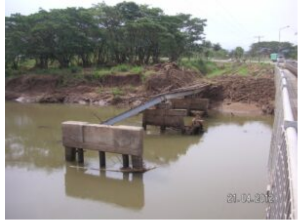
A tramline bridge bruised and battered by the April floods
