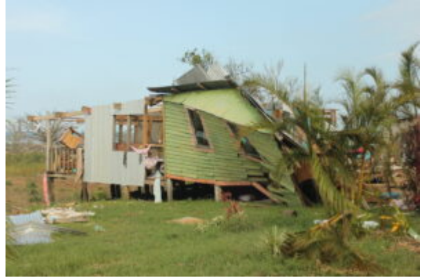
Damage caused by Tropical Cyclone Winston in Fiji in 2016
