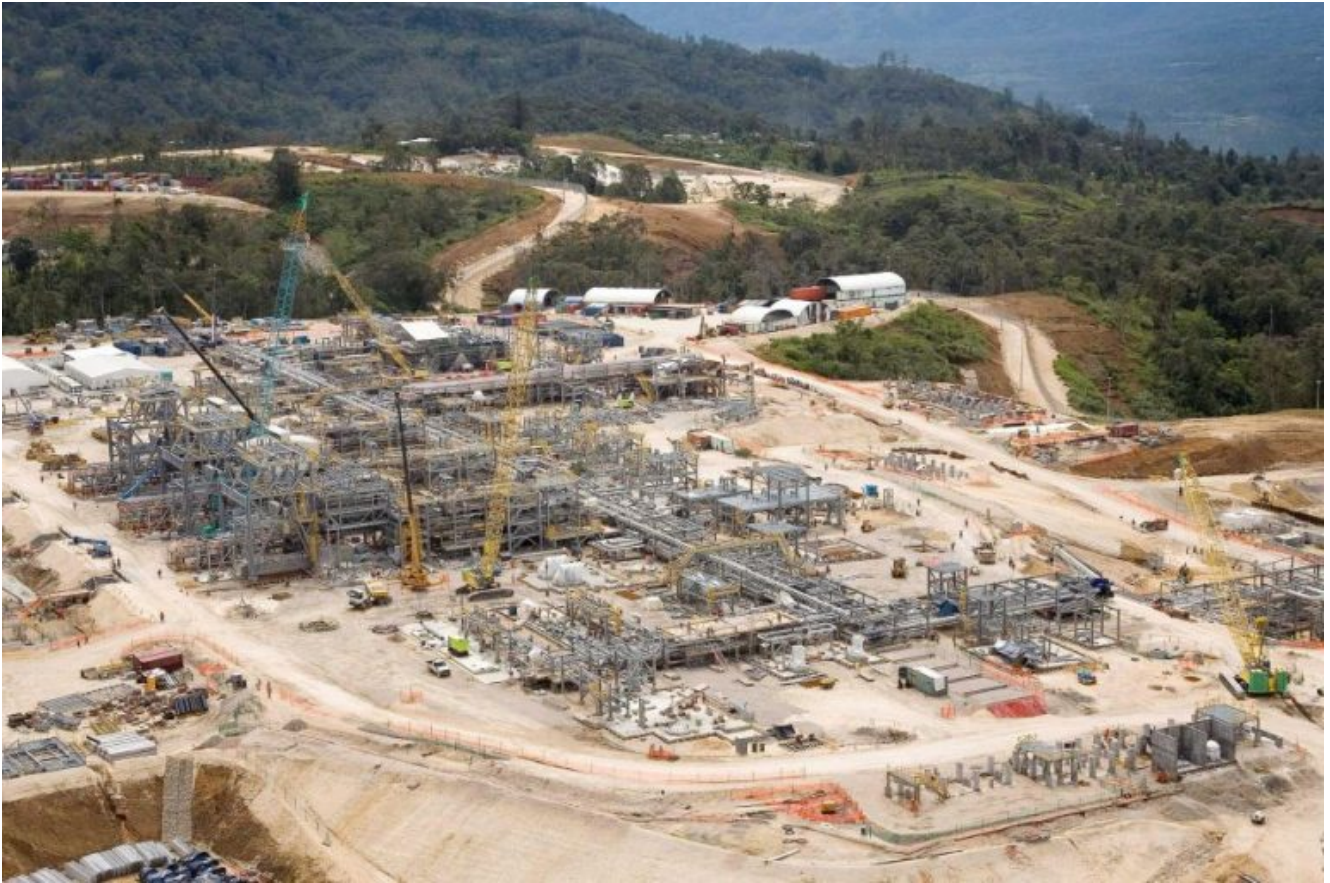
ExxonMobil LNG plant in Southern Highlands (Credit: ExxonMobil PNG)
