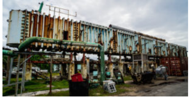
Abandoned infrastructure in the Pacific Islands Photo Credit: Asian Development Bank
