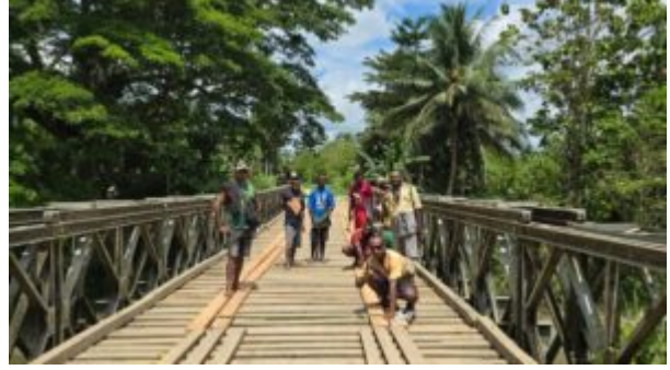
Local level government funded the repair of a bridge in North Wosera, East Sepik
