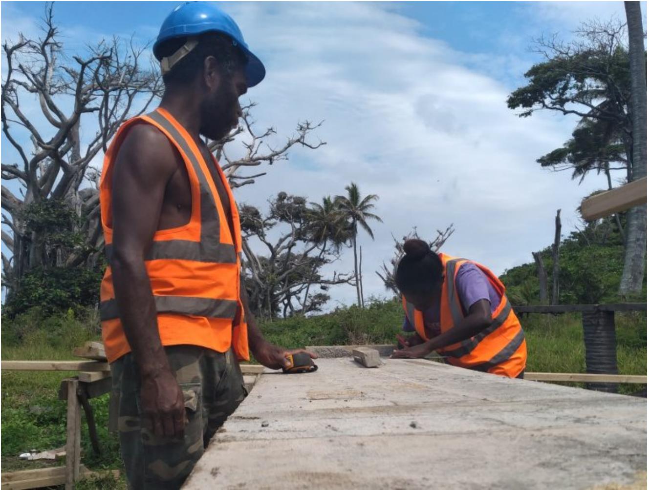
Trainees working on the construction of the Provincial Area Administration Office at Imlao village, South West Tanna (Fenda Sam)
