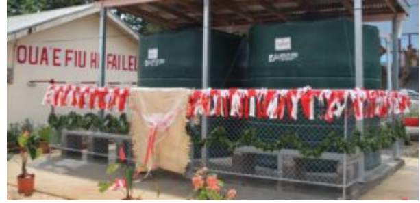
A newly-installed water tank at the Government Middle School, Nuku'alofa.
