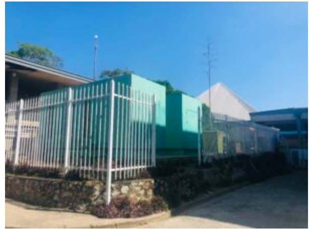
Standby generator at the University of PNG Photo Credit: Michael Kabuni
