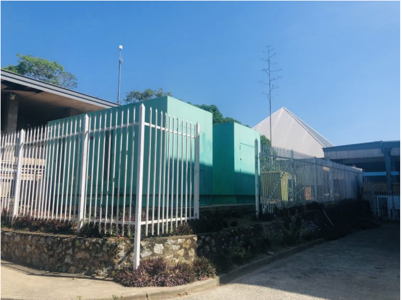
Standby generator at the University of PNG (Michael Kabuni)
