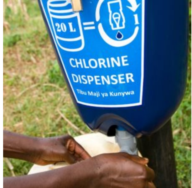
A chlorine dispenser installed as part of a randomised control trial in Kenya and Uganda (Jonathan Kalan/DIVatUSAID/Flickr/CC BY-NC-ND 2.0)
