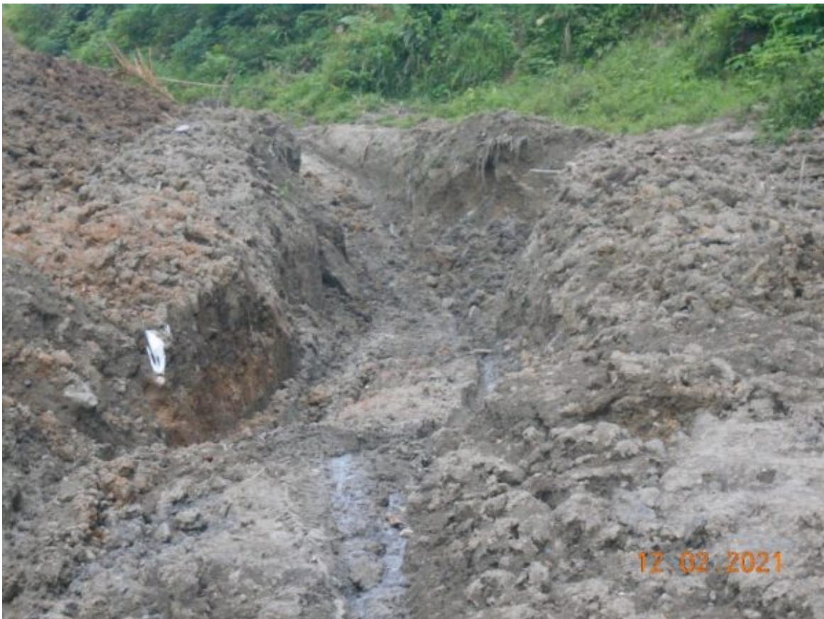
Worst section of the road from Lumi to Vanimo (Desmond Narongou)
