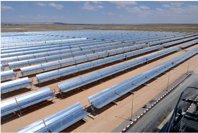
Thermo-solar power plant
